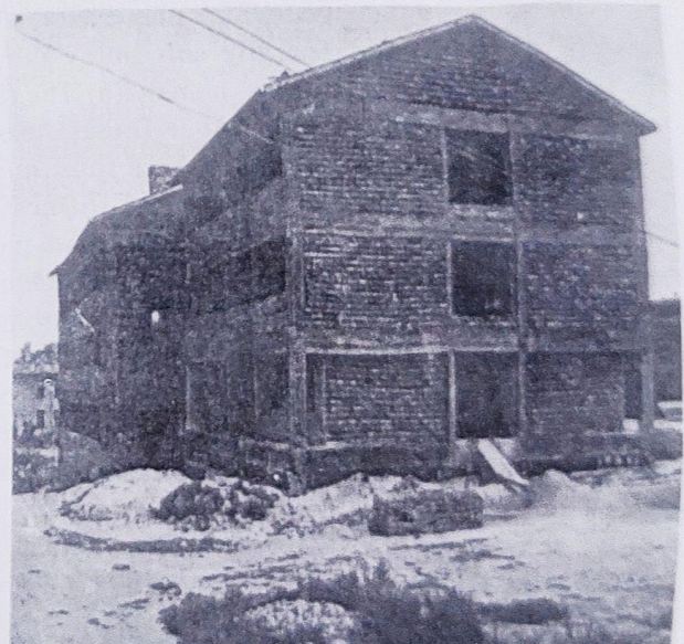
Fig.6: Under construction, across the street from Burdur's hospital, is this 3-storey school, of rather common design in Turkey. Every exterior column, between the top of the foundation wall and the bottom of the first floor, was shattered, causing the building to settle slightly. There was also minor damage to brickwork at roof level and in the first storey.
