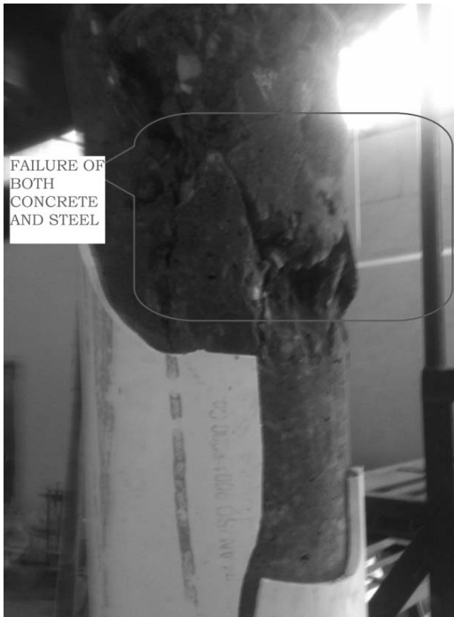
Fig. 6: Failure of both Concrete and Steel
